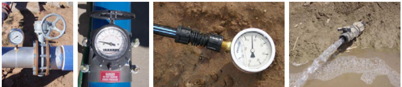
From left to right: Pressure gauge on mainline; flow meter; pressure gauge on tape; monitoring tape flush water.
